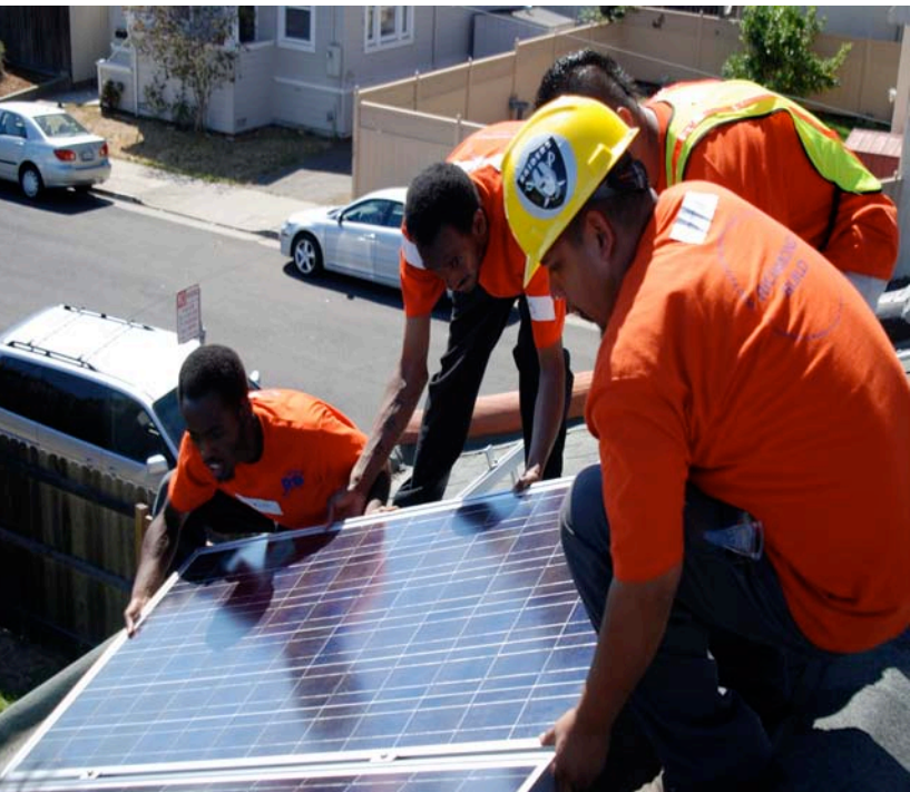
Photo courtesy of Solar Richmond, Richmond BUILD, GRID Alternatives, the Ella Baker Center for Human Rights, and greenjobsnow.com .
